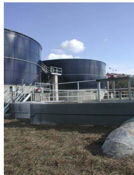
Image 1.29 Greater Hazleton Joint Sewer Authority Sewage Treatment Plant ( Source: Project Team).
